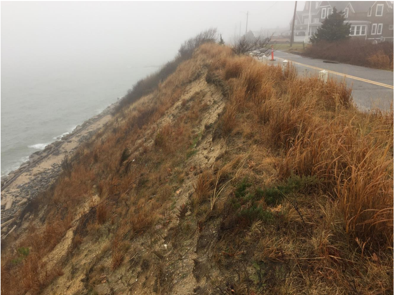
View South of the Failing Coastal Bank and adjacent roadway (Typical) in January 2017
