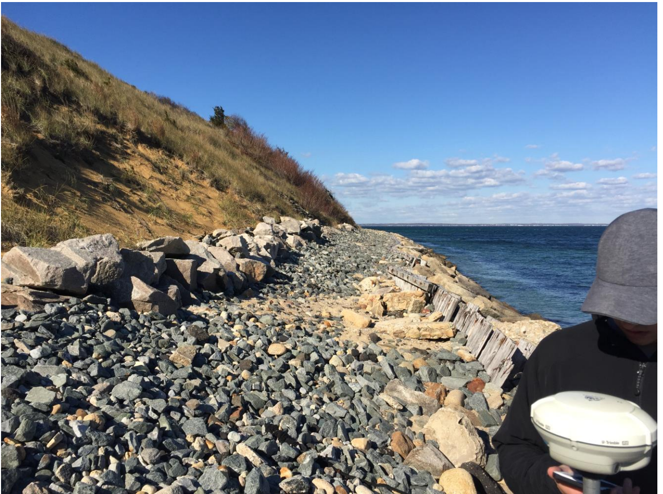
View North of the Deteriorated Stone Revetment & Eroded Coastal Bank (Typical) in November 2016
